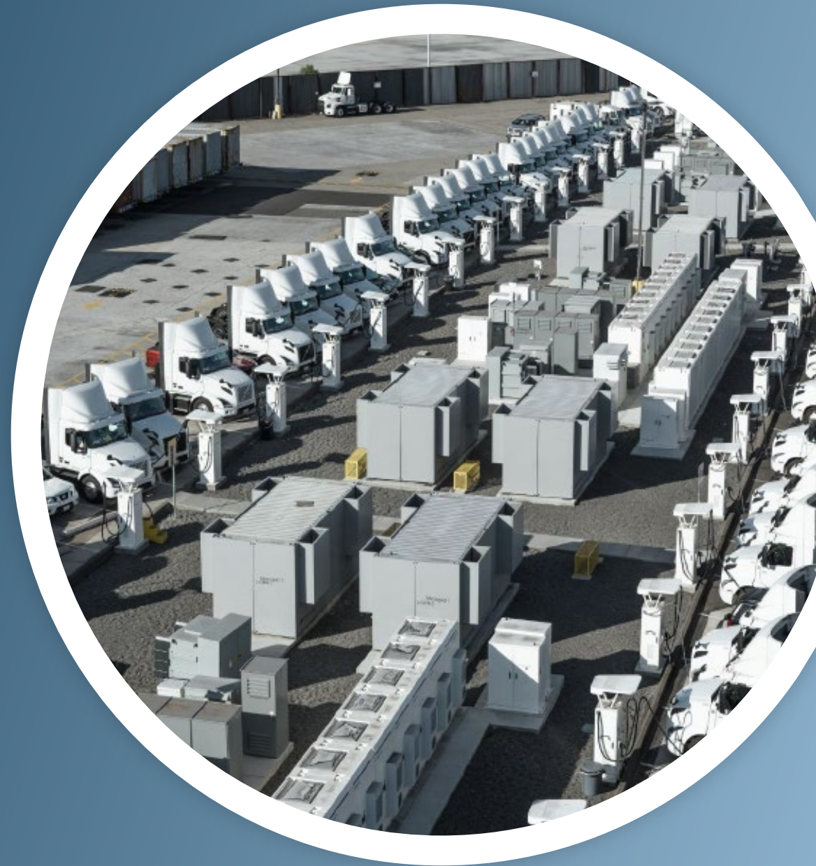
MICROGRID WITH 3 MW OF LINEAR GENERATORS for Prologis
